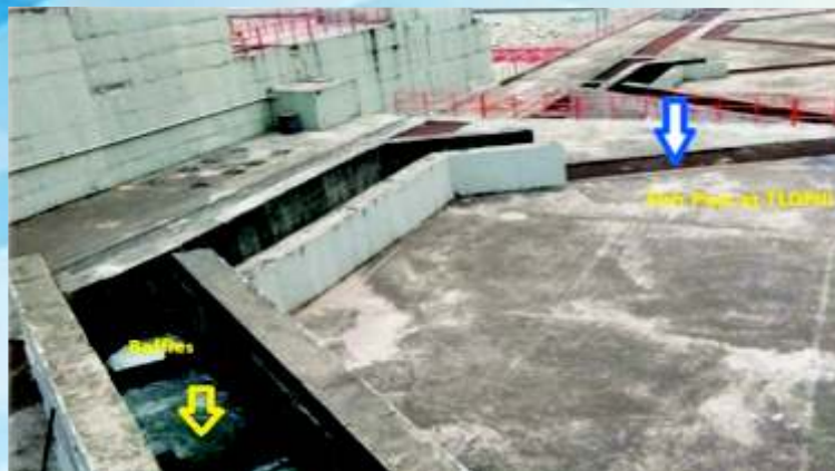
Fish pass structure at TLDPIII, Teesta
